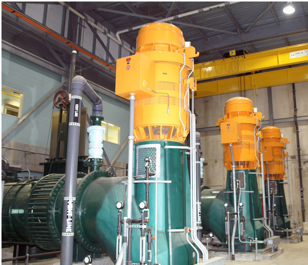
Pumping is a significant water production expense, particularly to deliver water to communities that are farthest from the treatment plants or at higher elevations. Electrical usage also increases during higher demand days in the summer.
